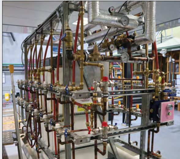
By plumbers for plumbers One of the custom-built TMV rigs built by NSG Plumbing
